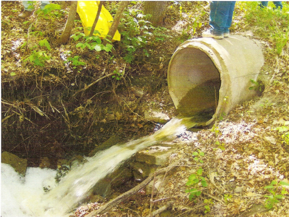
Photo #2 - Separated Culvert Just Downstream of West Alpine Lane
